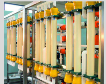
Ultrafiltration - Highly Purified Water Ultrafiltrationsbank - Highly Purified Water
