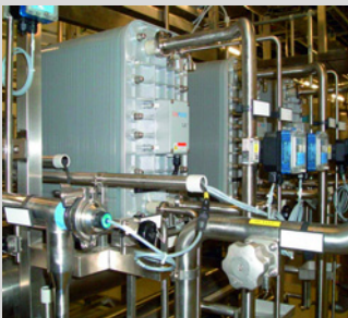
Electrodeionisation - Purified Water Elektroentionisierung - Purified Water
