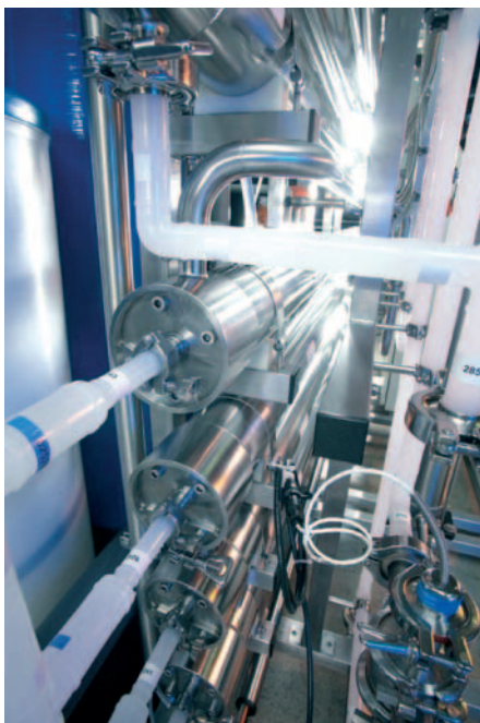
Abb. 1: HPW Highly Purified Water System 600 l/h
