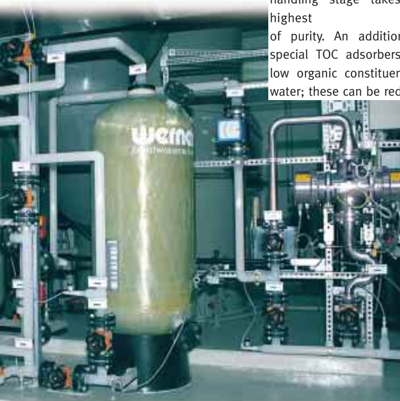
UV oxidation, polishing stage and 0.1 µm membrane filtration (15.000 l/h)
