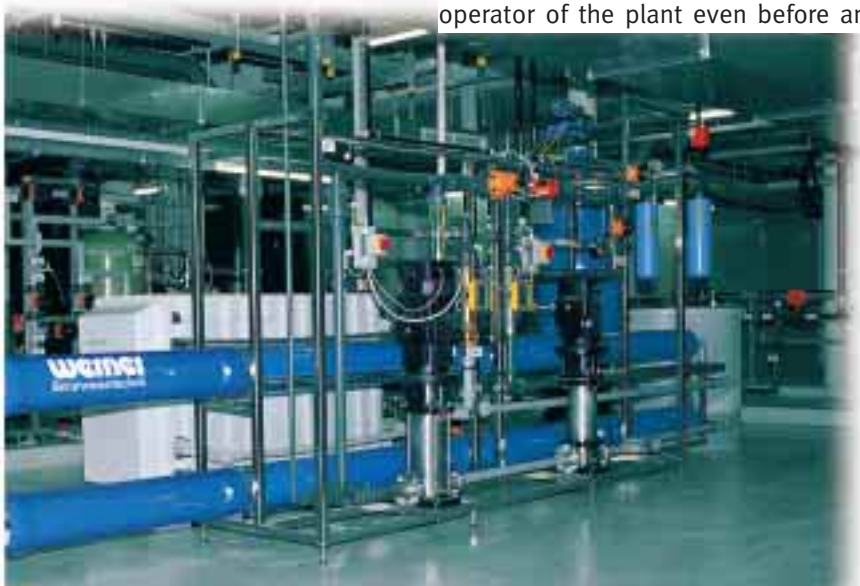
WERNER reverse osmosis plant for the micro-electronic industry
